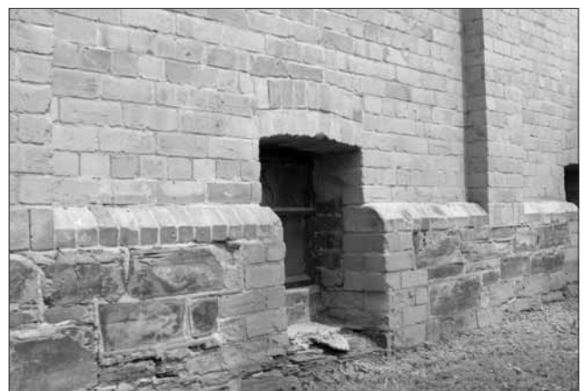
BELOW: 1883 – 1901 The north wall of the kindergarten which contains engravings by the boys. Details of the brickwork engravings appear opposite.
